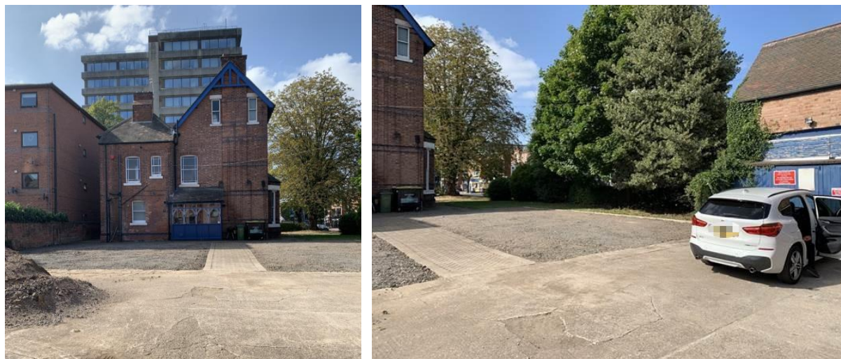
Work in progress to create ample car parking space for a variety of uses
